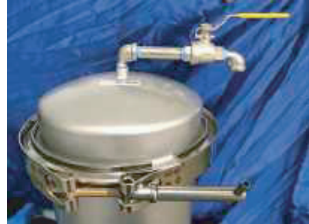
Air Purge / Relief Valve
