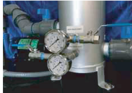
Pressure Gauges & Drain Valves
